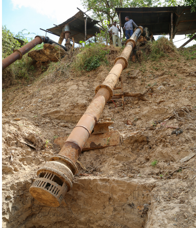
Residents of Shukurow village in Somalia examine damaged local irrigation systems. CRS is working in these regions to aid families affected and uprooted by the drought. Photo by Mohamed Sheik Nor for CRS
