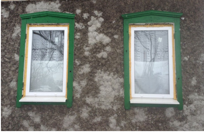
New windows in Popasnaya. Before receiving assistance, the house was non-heat-efficient and cold. At the moment, Alexander Vasilievich feels much more comfortable, thanks to the opportunity to restore the heat in his home.
