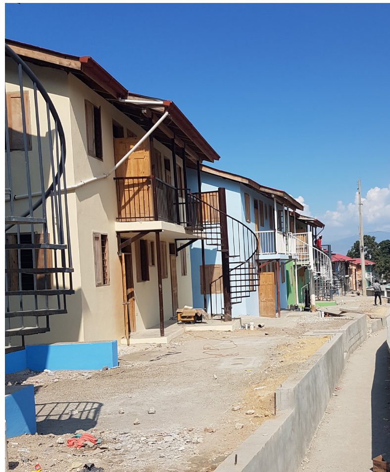
Permanent housing and community infrastructure along main road. Photo: Gesner DeVilmar / CRS
