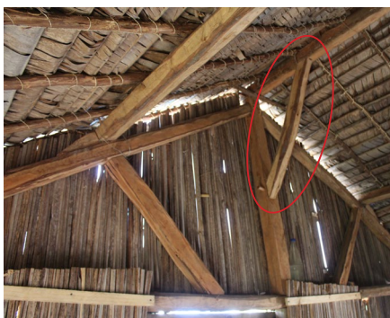
Wood trusses are reinforced with a diagonal bar attached to the top rafter.
