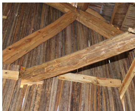
The top frame and beams are structurally stabilized by introducing horizontal reinforcement bars in the 4 top angles.
