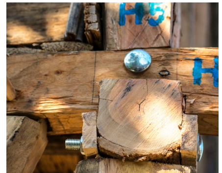
The connections of the four main stilts of the cross-bars that support the stilts of the superstructure are reinforced with bolts.
