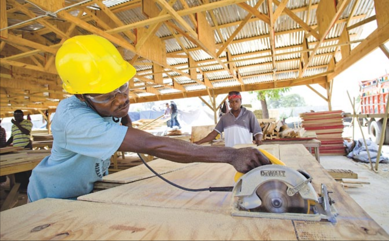
You help Haitians rebuild their own communities. Carlos Loresilien was hired by CRS to build temporary shelters as part of a partnership with a factory in Port-au-Prince. Photo by Benjamin Depp for CRS
