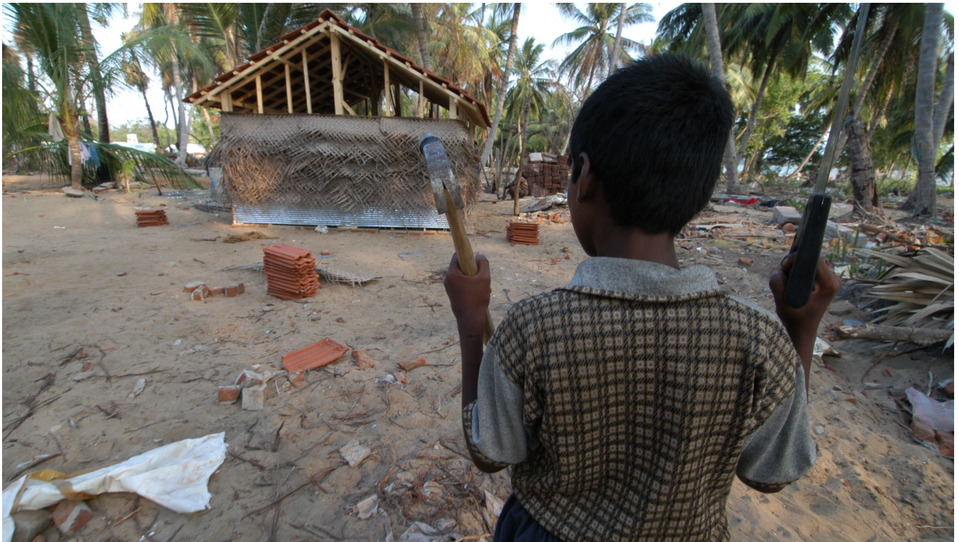
Prakash fetches a hammer and a saw to help his father finish the walls of their temporary home, provided by CRS/Caritas.
