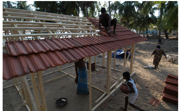
Workers labor to roof a CRS/Caritas provided temporary shelter in Navalady, one of 86 such homes provided by CRS/Caritas in the community, which was nearly wiped out by the tsunami. In all, the roof consists of 400 clay tiles, each costing about .14 cents, which help to keep the insides of the homes cool in temperatures exceeding 100°F (38°C) in the hot months.
