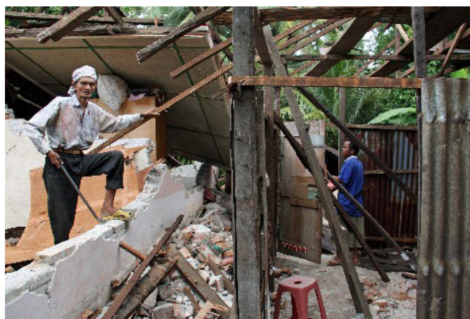
Over 1.25 million people were affected by the earthquake and over 135,000 homes were severely damaged
