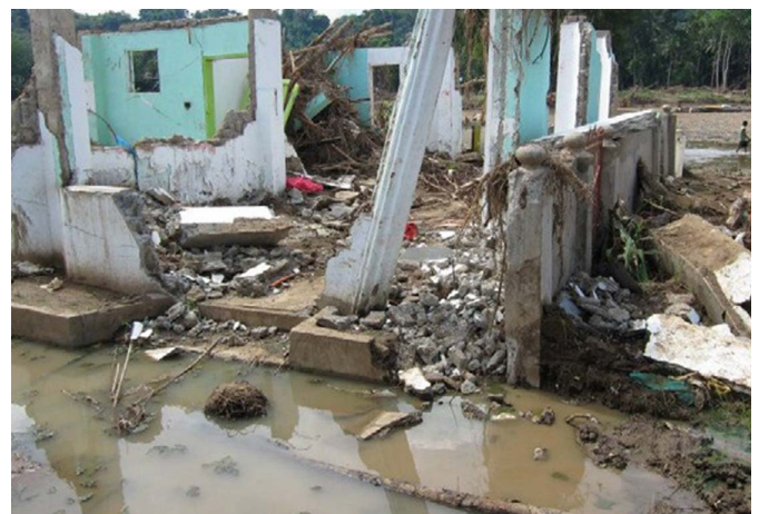
Extent of damage caused to dwellings due to the storm. Photo: Charisse Mae Borja / CRS
