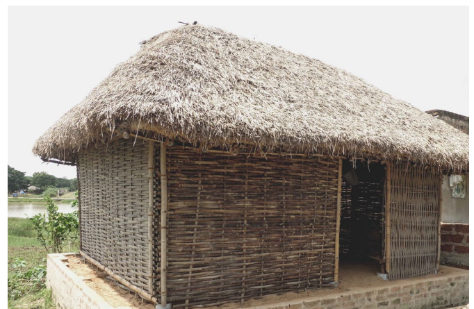
The woven split bamboo mesh walls are then mud plastered inside and outside, once the hipped roof is completed
