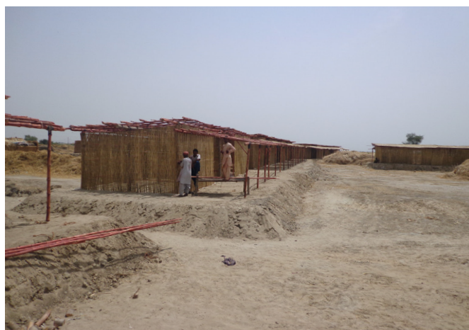
Building shelters on a raised plinth is one of the most effective ways of reducing damage to shelters during flooding. Drainage ditches were dug with stone or earth curbs dug around the perimeter of shelter to divert rainwater away from the house. A small number of non-beneficiary households replicated the technique when building their own houses.
