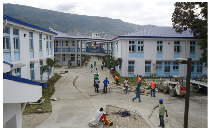
Workers make the finishing touches to the hospital grounds before handing over for opening. Photo: CRS
