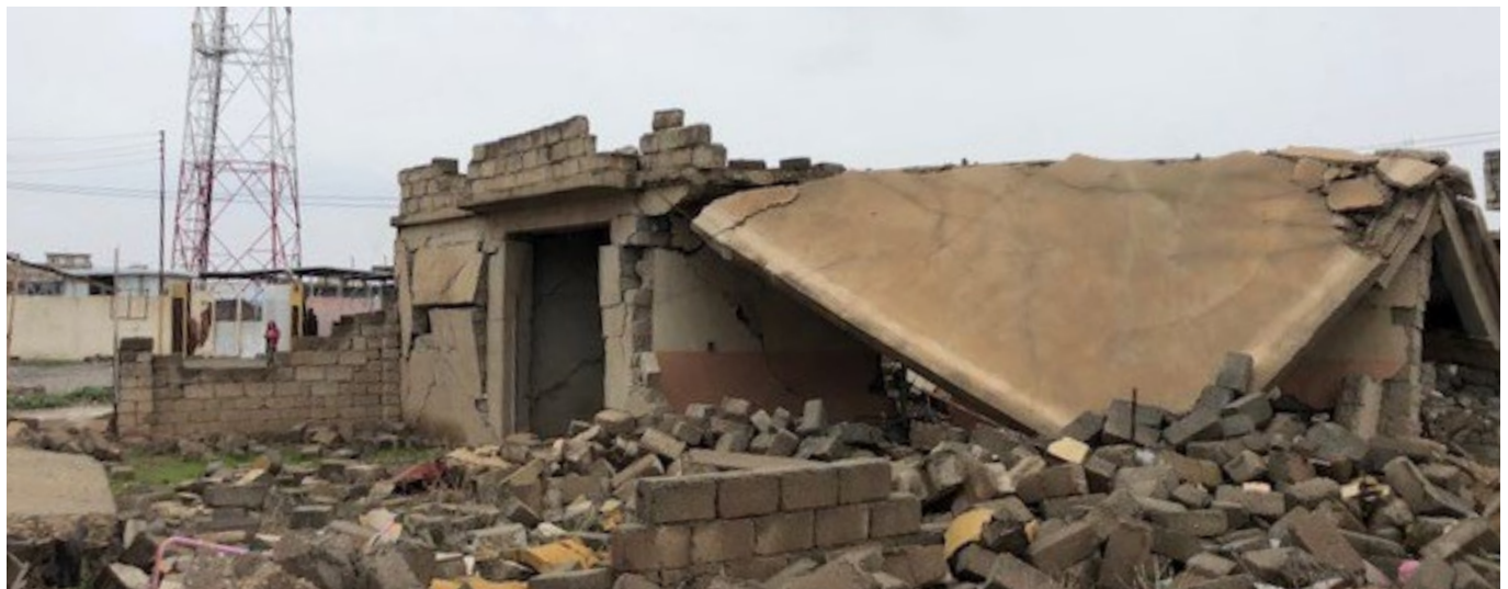
Totally damaged house in Kharaba Sultan village of Ninawa, Iraq. Photo: CRS
