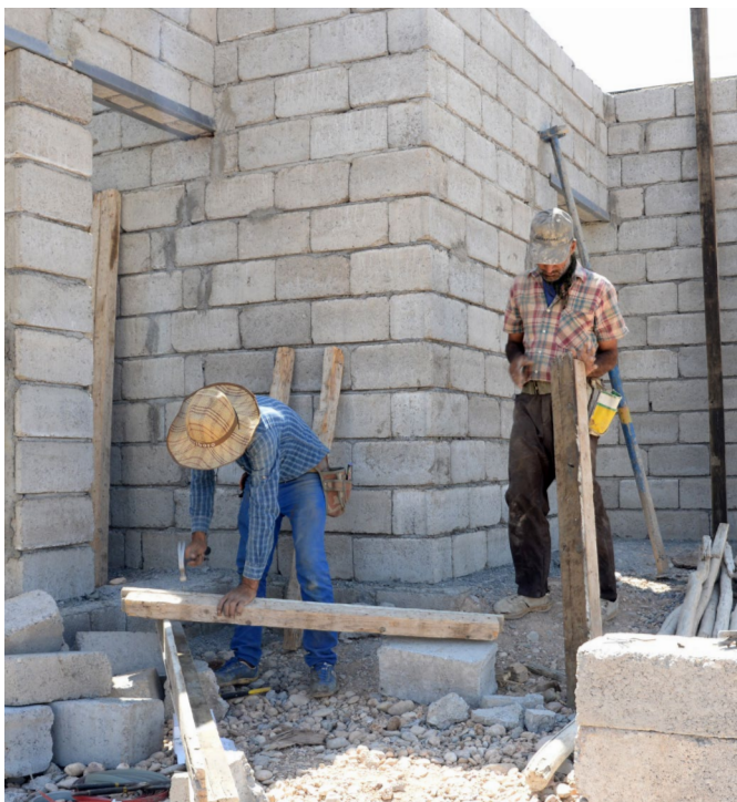
Building walls and molding for reinforced concrete roof of the core housing unit in Tobzawa village of Ninawa, Iraq.
