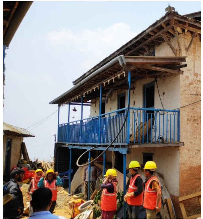
Ward No. 5, Temal Rural Municipality, Kavrepalanchok: Demo retrofit house carried out as part of the DFID funded retrofit project implemented by a consortium of UNOPS, Build Change, and BBC Media Action. Two male and three female masons are being trained under two head masons and an engineer.
