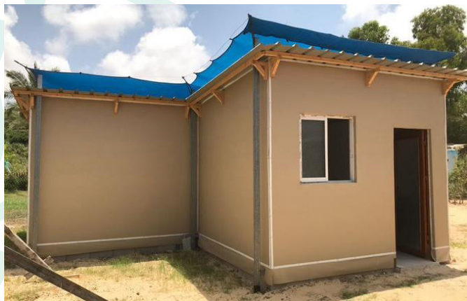
1st place design (top) and construction of the 1st place design (bottom). Photo: CRS
