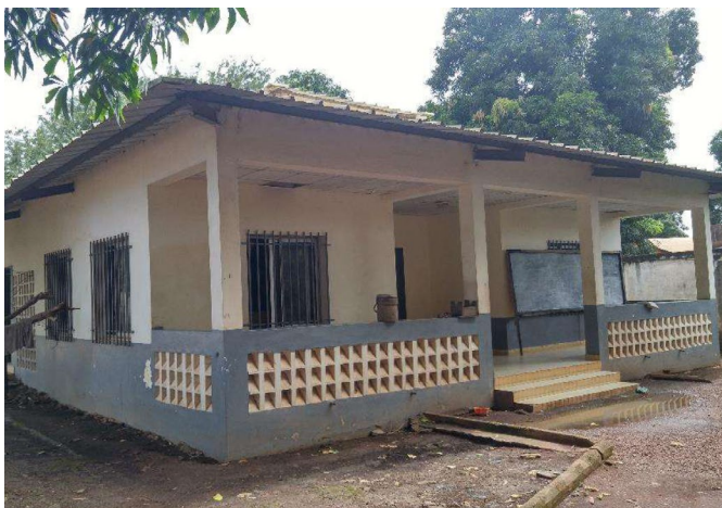
Housing facilities (roof leaking, damaged ceiling, non-functional toilet and without perimeter slab), Kankan, before.
