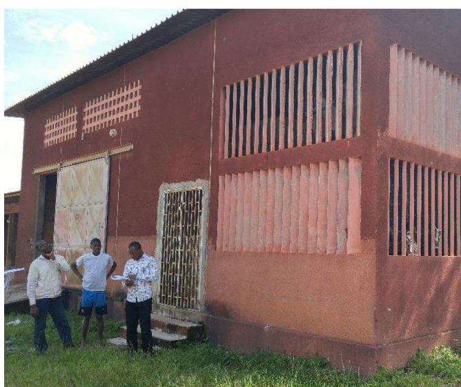
Epidemiology Warehouse (Rain water is passing through the wall air slots. Demolish air slots concrete and install permanent windows with security grilles. Provide ramp to access stock room #2), Labé, before.
