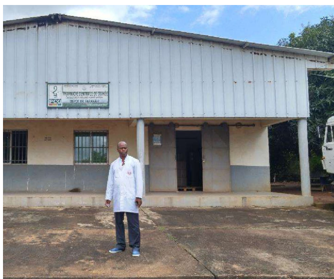
Main Warehouse (Deterioration of roof, ceiling, doors & locksets, paint on walls), Faranah, before.
