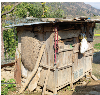
Earlier goat shelter design. The lack of ventilation and drainage resulted in unhygienic conditions that led to disease among the goats. Photo by Jennifer Hardy/CRS
