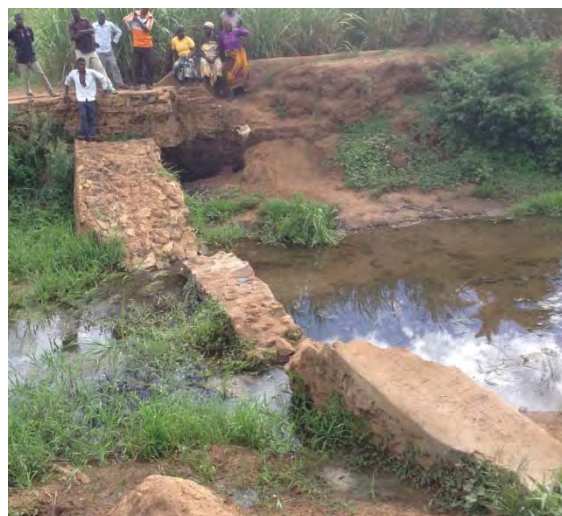
Photo 5. Natama Weir Failure
