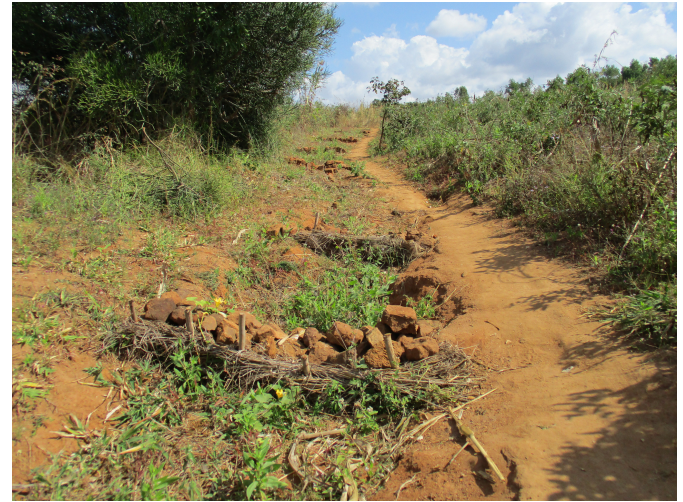
Figure 1: A series of check dams run perpendicular to a well-traveled path and have been successful in filling the gully in with sediment.
