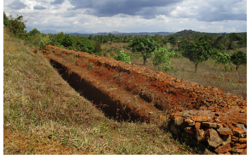
Figure 1: A water absorption trench surrounded by a stone bund acts as a water overflow catchment barrier at the bottom of a large slope but above farmer's agricultural fields.
